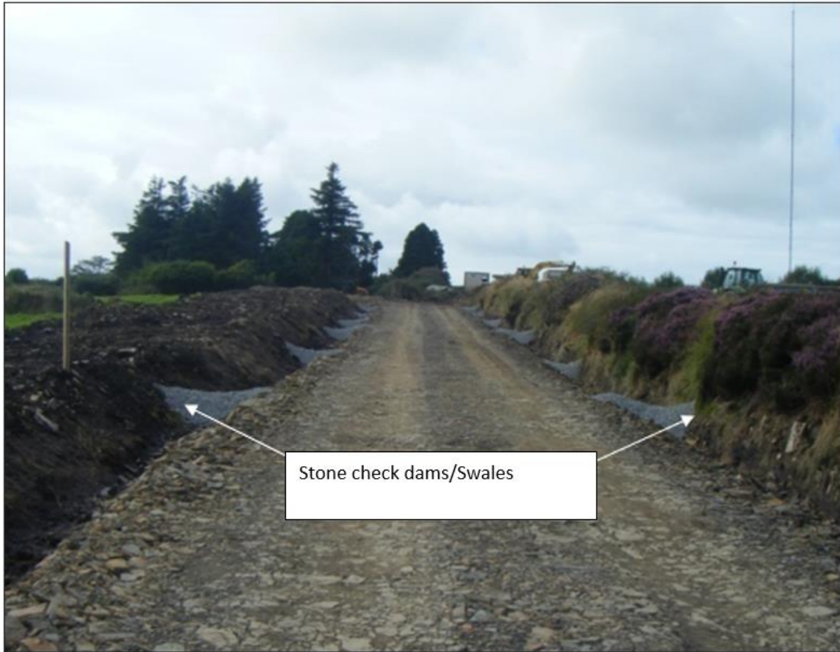
Figure 3-21: Examples of check dams along access track drainage channels
