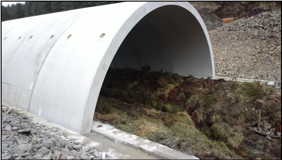
Figure 3-14: Typical clear span pre-cast concrete arch units in place over an existing watercourse
