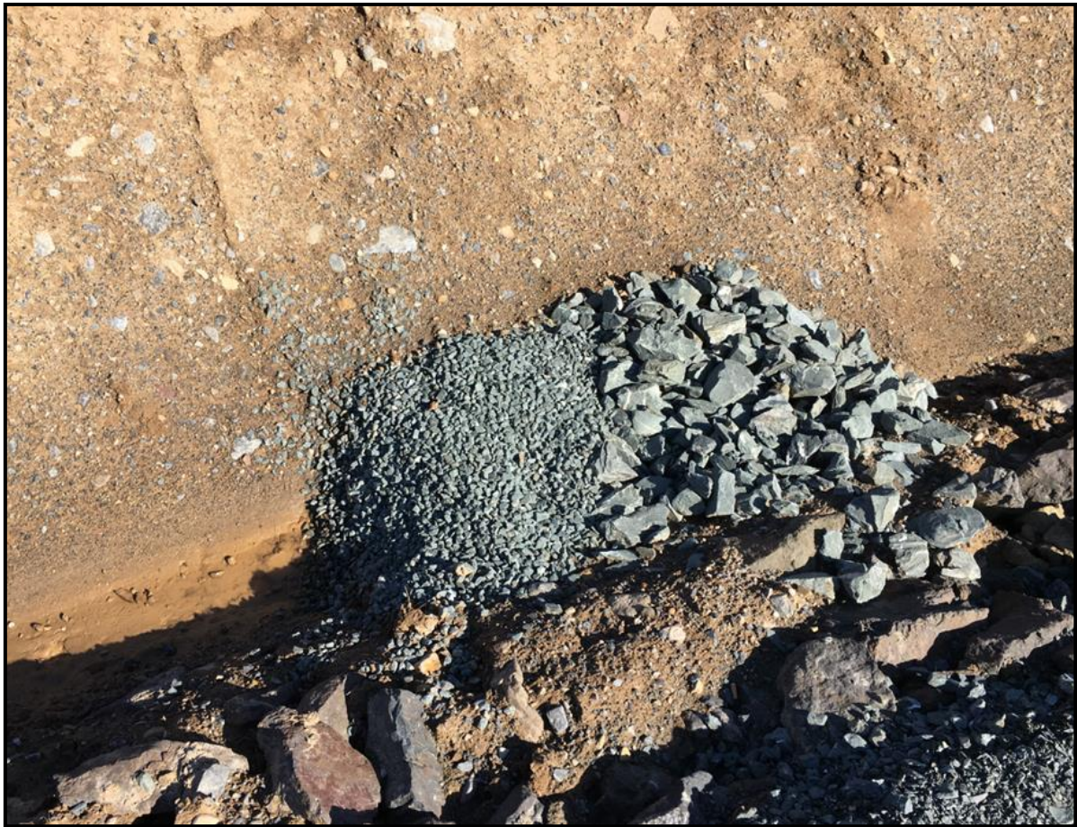
Figure 3-19: Stone check dam with large aggregate on downstream side
