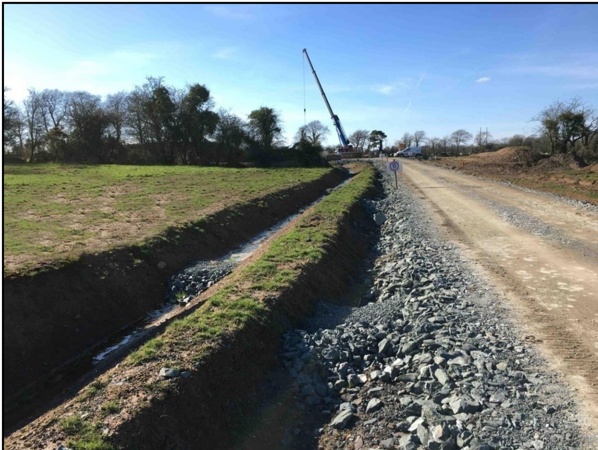
Figure 3-13: Separation of Clean and Dirty Water Drainage on A Wind Farm Site
