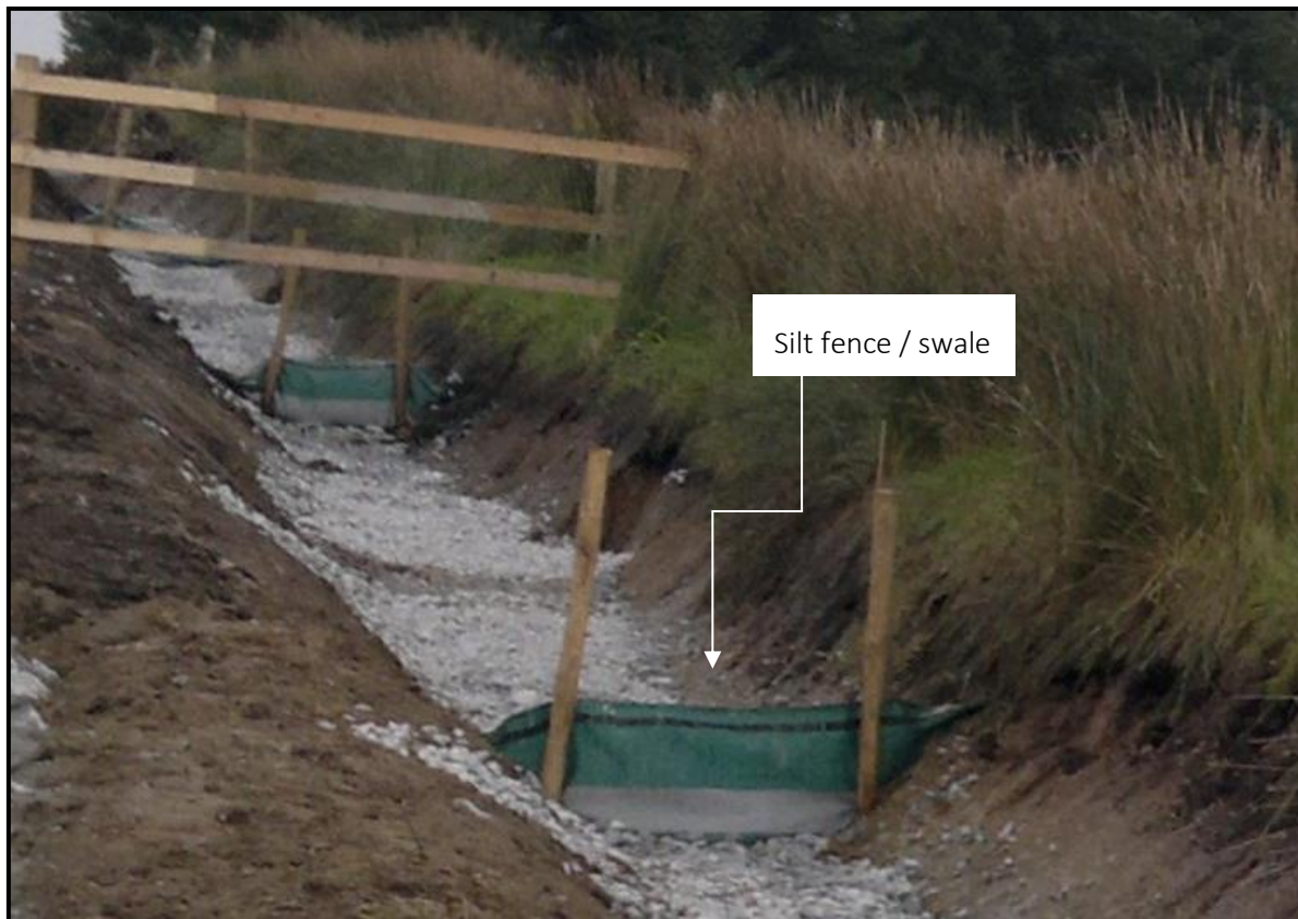
Figure 3-22: Example of a silt fence used in conjunction with check dams along access track drainage channels
